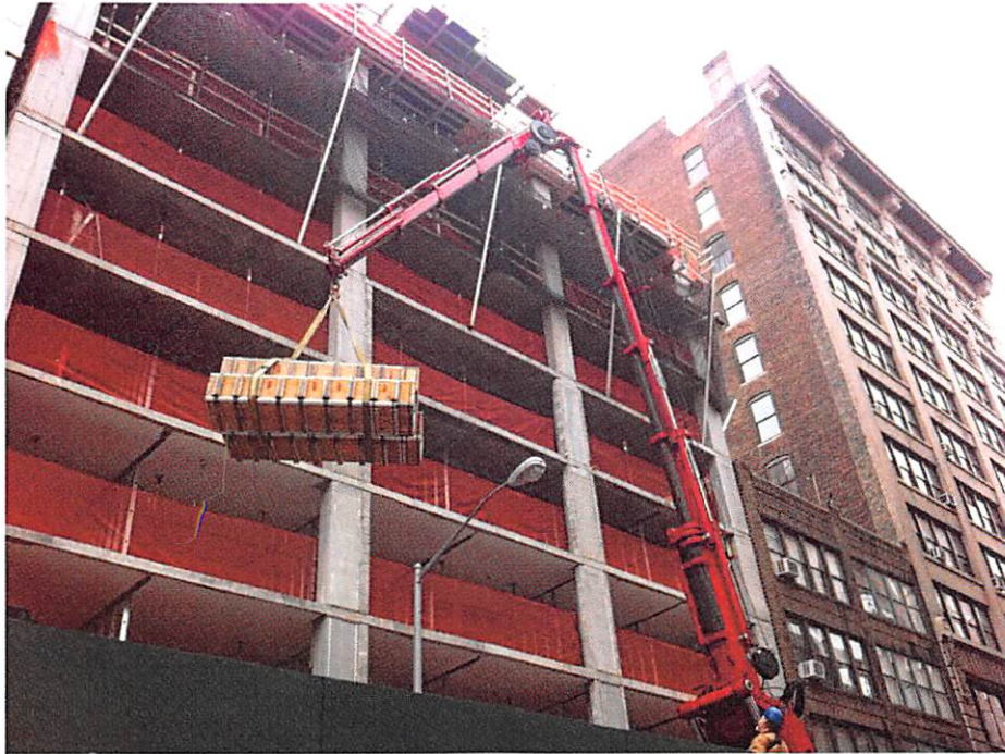
Method #1: Columns are lifted to position and dropped over the Rebar cage from the floor above. West 21 st Street, NY, NY
